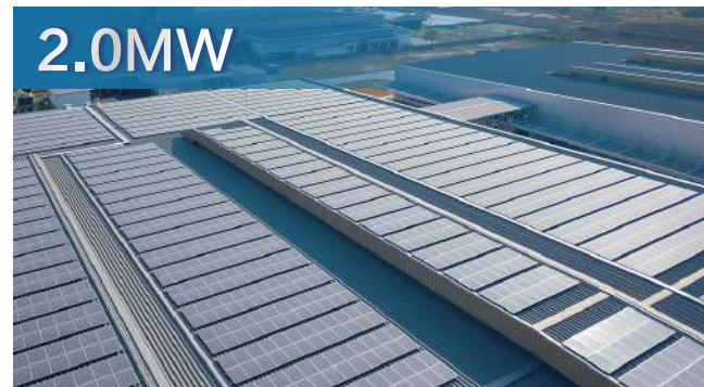
PROJECT | Weishida rooftop distributed PV power station
