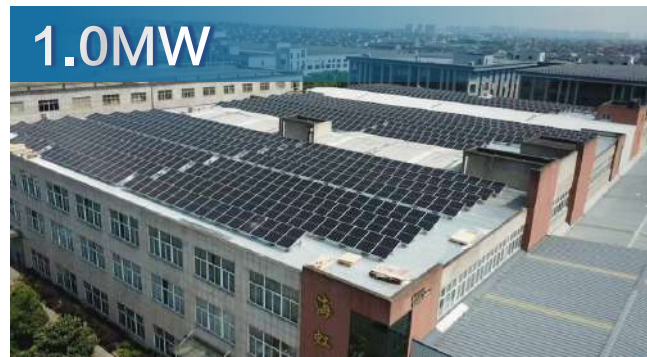
PROJECT | Ningbo Haihong rooftop distributed PV power station
