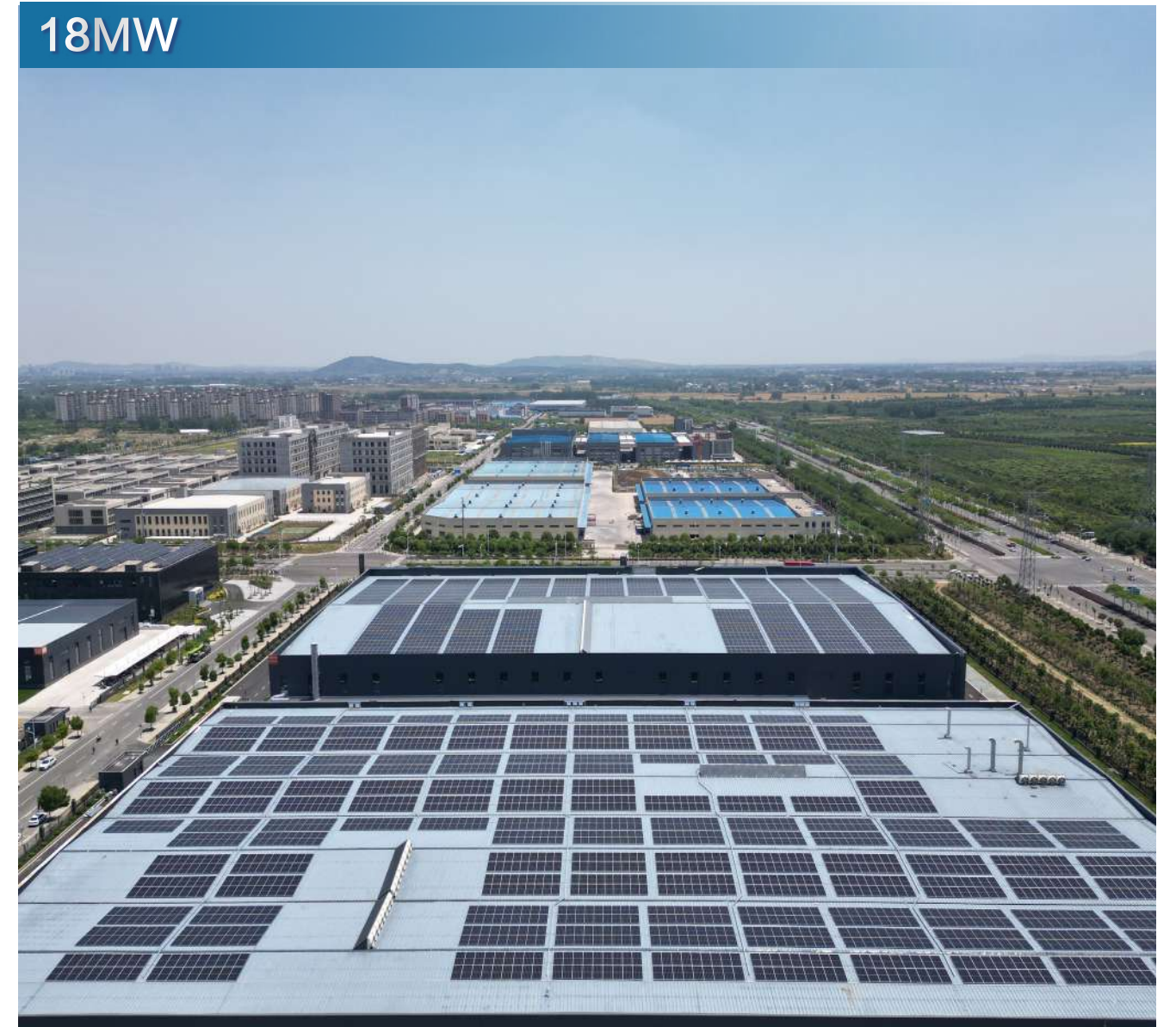
PROJECT | KMNMT rooftop distributed PV power station
